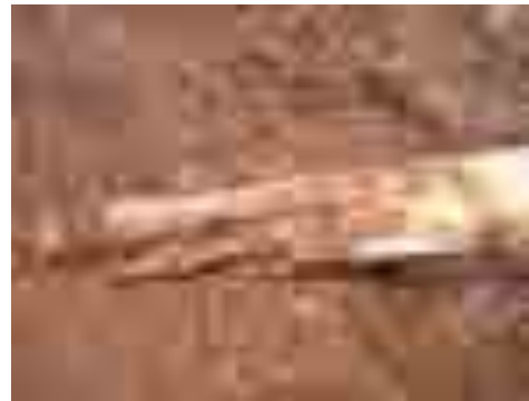
Foto 7: Ataque de termitas Photo 7: Termite attack
